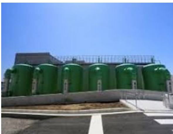
D. Advanced Technology of Water Circulation Kawai Purification Plant
